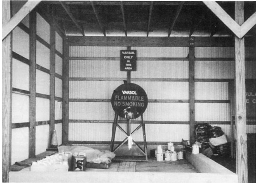
Provide Secondary Containment For Chemical Storage
