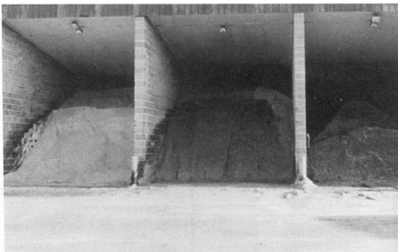
Cover Potential Pollutants Such As Sand And Salt If Possible.
